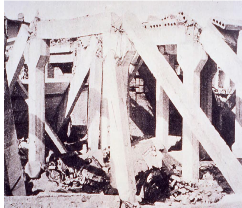
Unseating of precast concrete beams off corbels of columns ( fib 43 )
